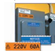
Electrical Panel Identification
