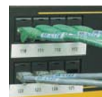
Patch Panel Identification
